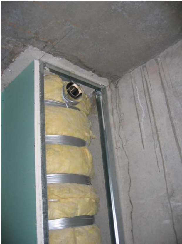
Picture 3: Concrete cork, mineral wool insulator, metal support of the sheathing and the sheathing made of drywall panel
